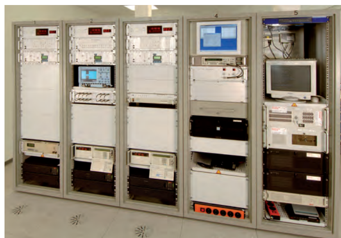
Figure 8: DCF77 control facilities of PTB. The atomic clocks, the drive signal generators and the electronic converters are installed in the racks 1 to 3. Rack 4 contains the local measuring equipment and the interface for communication between Mainflingen and Braunschweig. Rack 5 contains the interface for feeding in alarm and weather information.
